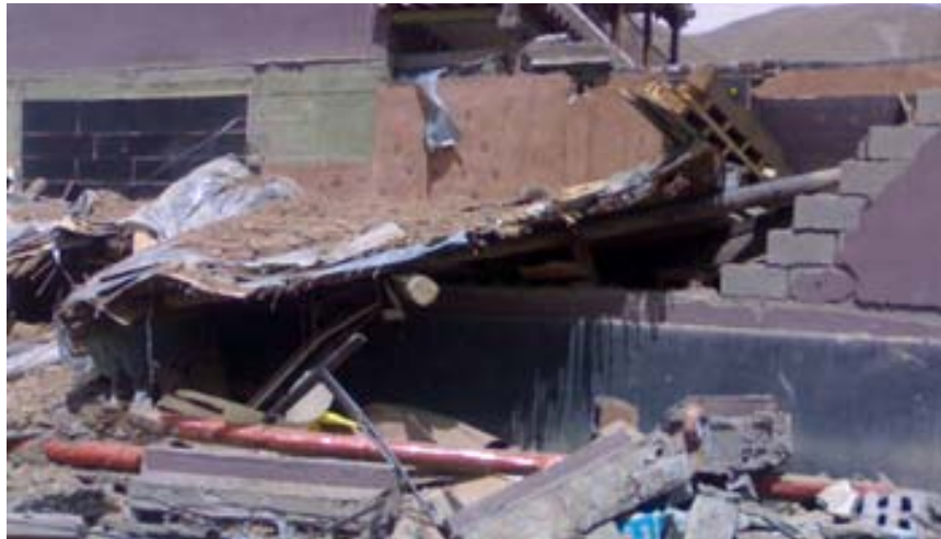
Many buildings near the epicentre were wrecked and access to basic utilities remain cut off in the aftermath of Wednesday morning's earthquake in Qinghai Province. Photo: Xinhua News
